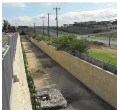
US 281 Concrete Stormwater Vault
